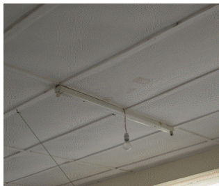
Poor electric lighting on wards
