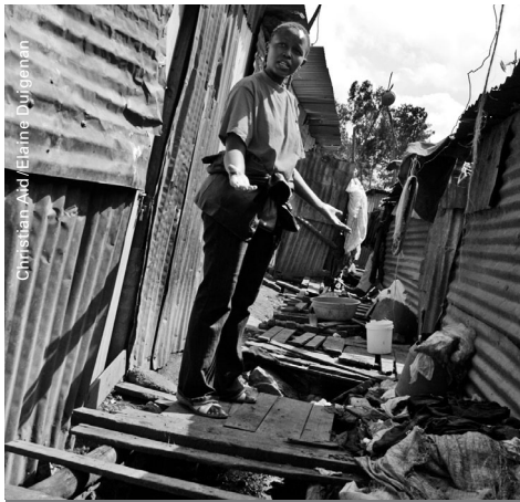
Catherine Kithuku shows the broken walkway over her community's drainage
